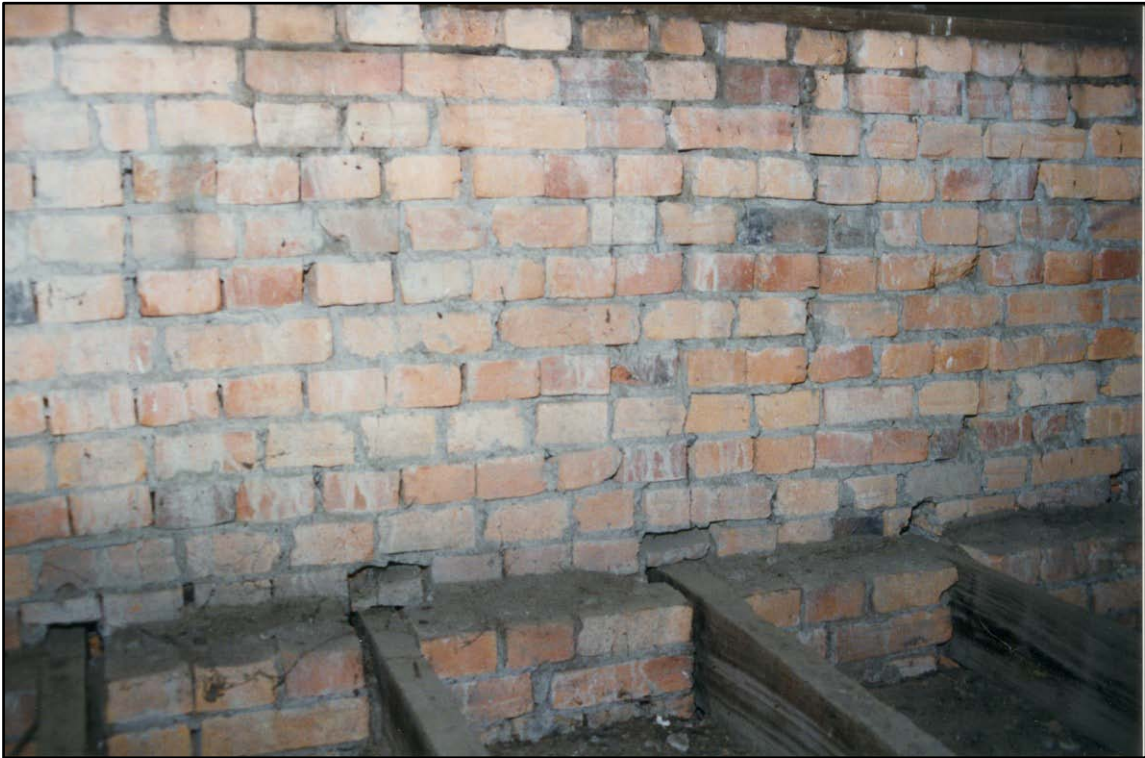
Photograph 12 Limey wash appearing on these loft wall above the north room and on the double flued chimney are likely the results of rain washing wet mortar during construction; above north room, and hand-sawn ceiling joists inserted into walls.
