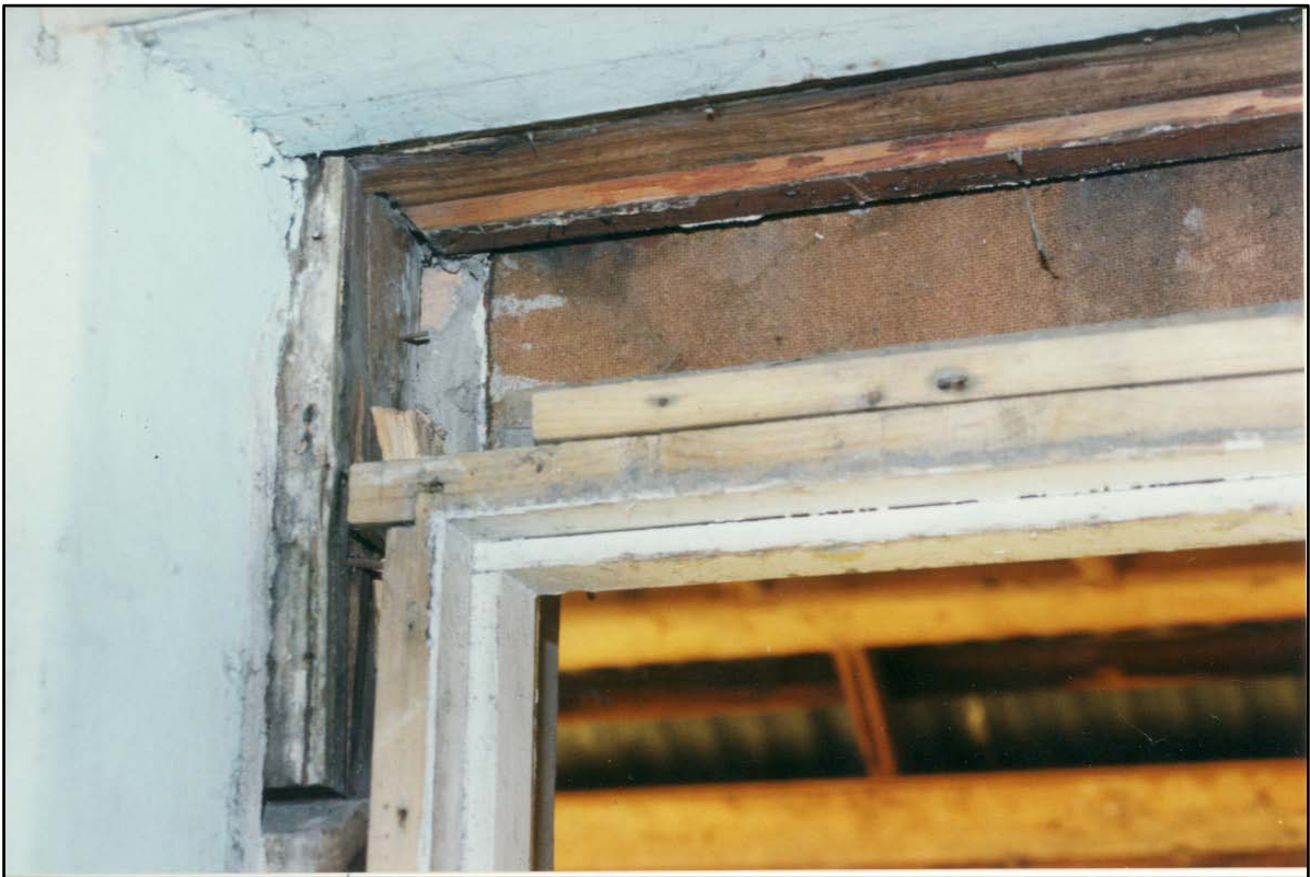
Photograph 17 Detail of transom light frame, front door, with modern door frame representing alteration. A decorative architrave in a pale yellow paint is partially concealed by the lintel in the opening.
