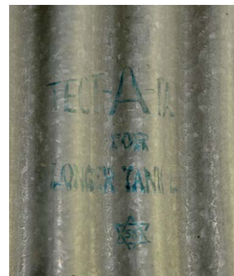
Photograph 39c March 2014. No date. Manufacturers mark on CI sheet.
