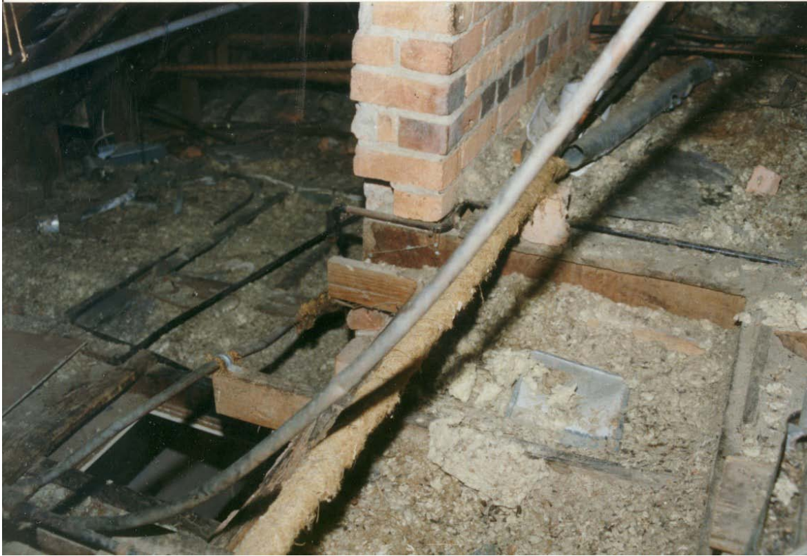
Photograph 70 Entrance way through ceiling to loft. entrance to side loft , lower left. The brick loft wall is seen centre and central loft is to the right.
