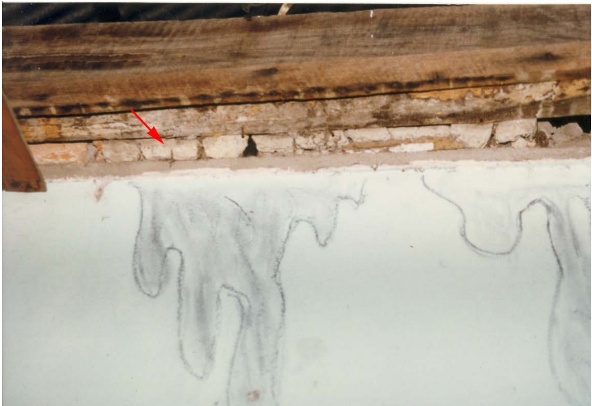
Photograph 19 Remnants of first ceiling plaster (arrow), in situ , caught between ceiling joists and wall, central room, Pontville, S2.
