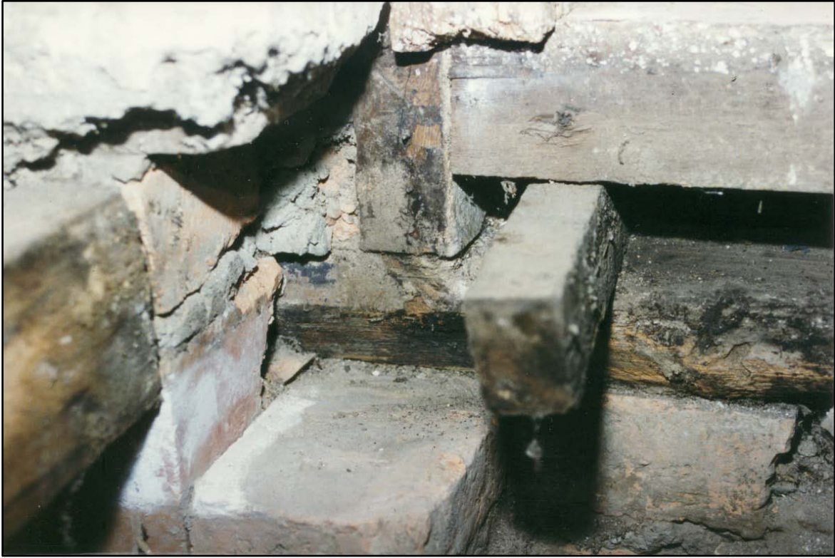
Photograph 16 Detail of base of the front door jamb assembly with moulding removed and showing hand-sawn hardwood timber, with modern sill at top. Former sill resting on bricks indicates original floor height.
