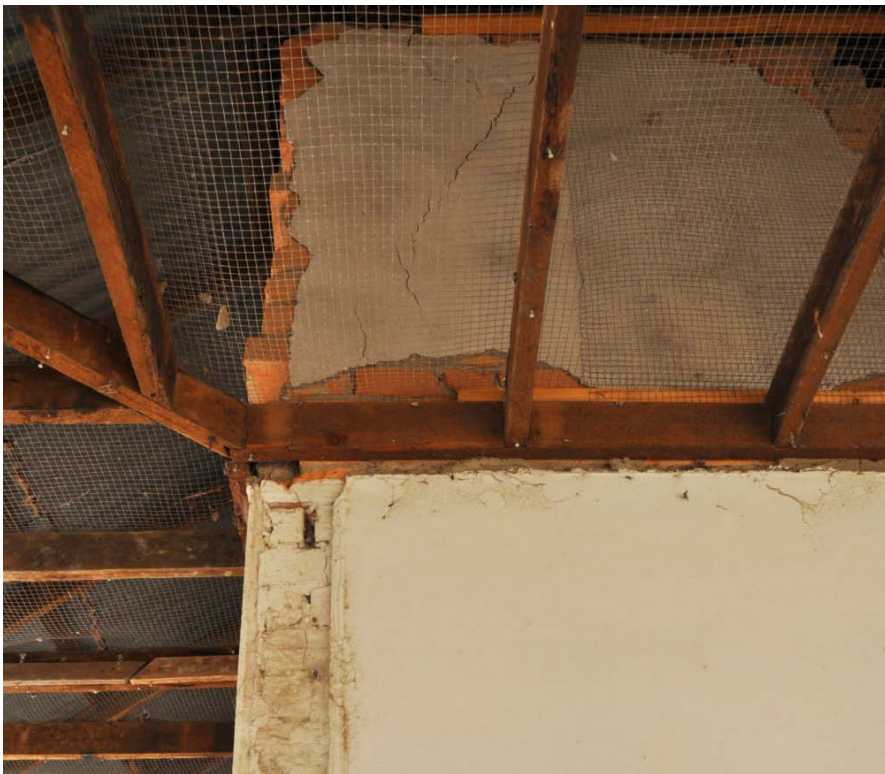
Photograph 25 The exterior bricks of the double leaf south room seen here from the end room project well beyond the vertical wall at staggered spaces and are covered by render.
