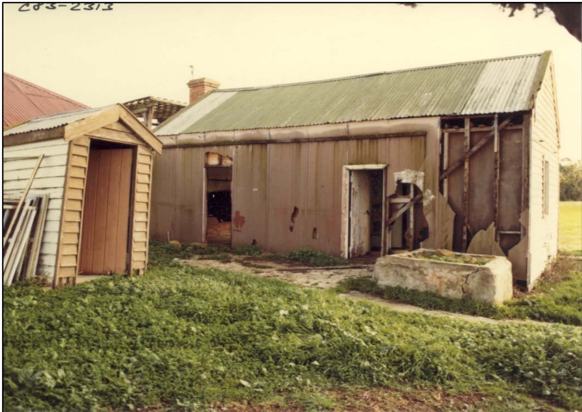
Photograph 37 The kitchen in the early 1990s well after abandonment, with some evidence of vandalism. The horizontal stripe over the doors may relate to a skillion roof, as observed by G. Hawthorne.
