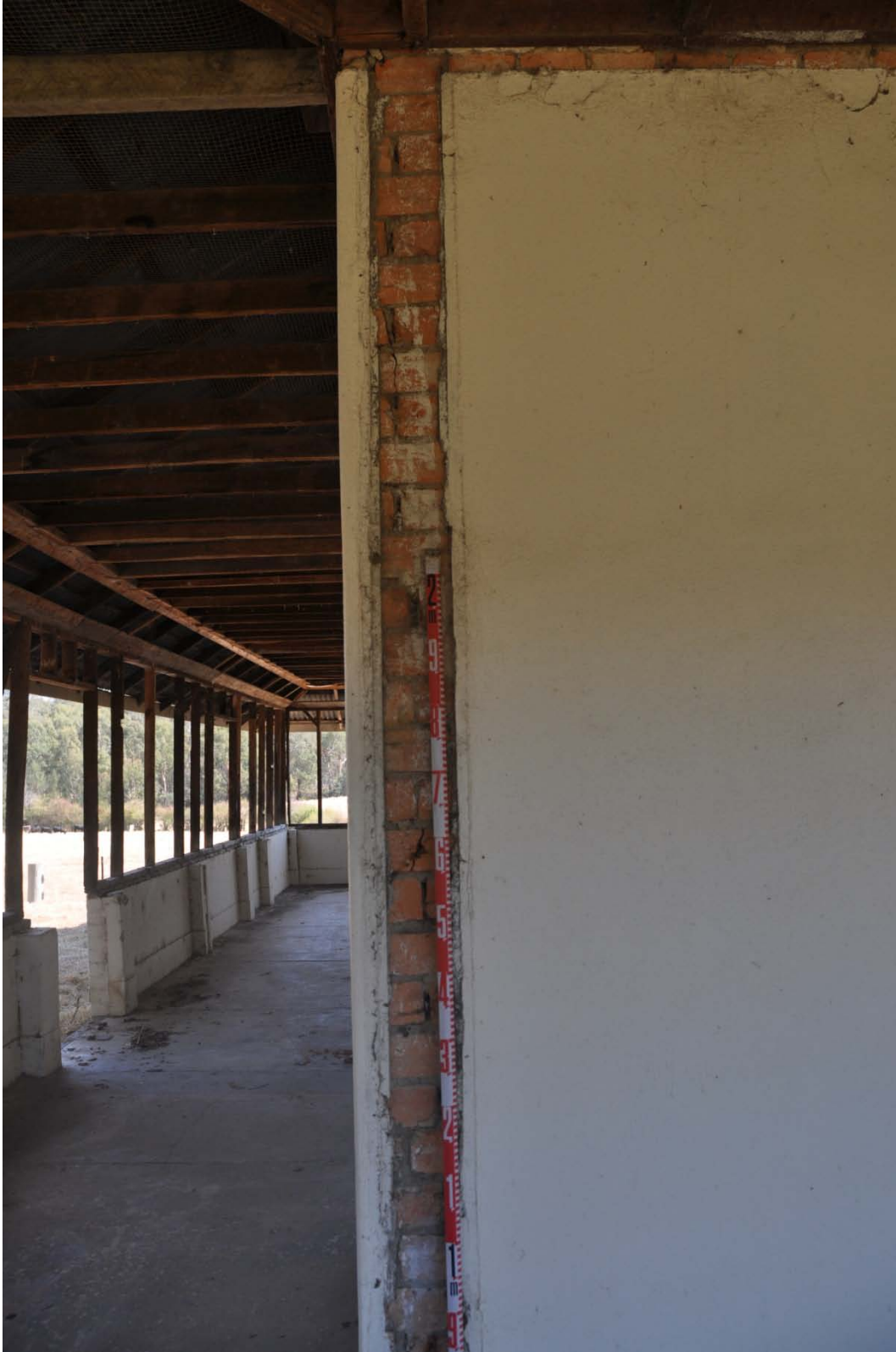
Photograph 26 Seen here is the southwest corner of core rooms showing repair to create a corner in the 1950s. Staggered vertical placement of bricks and the absence of full half bricks at this corner indicate that it is a renovation and was not ever a corner. A "hard" mortar covers this renovation. Scale 20 cm intervals.
