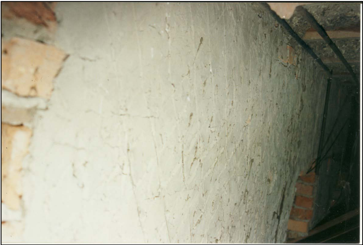
Photograph 71 The plaster on this vertical wall above the front verandah ceiling has been scored for a finishing coat.
