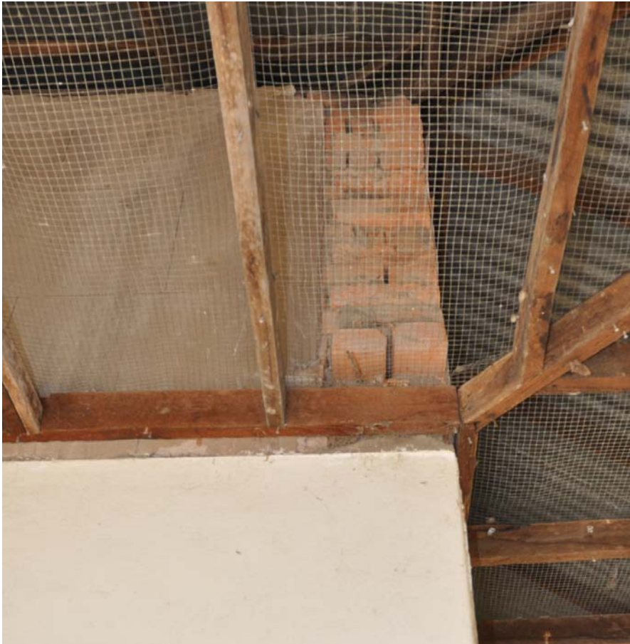
Photograph 24 The bricks of the double leaves of the south end wall seen here above the ceiling timber project beyond the vertical wall and are smeared with mortar on their vertical ends. Darkened ashlar lines are visible in the grey render of the loft wall.
