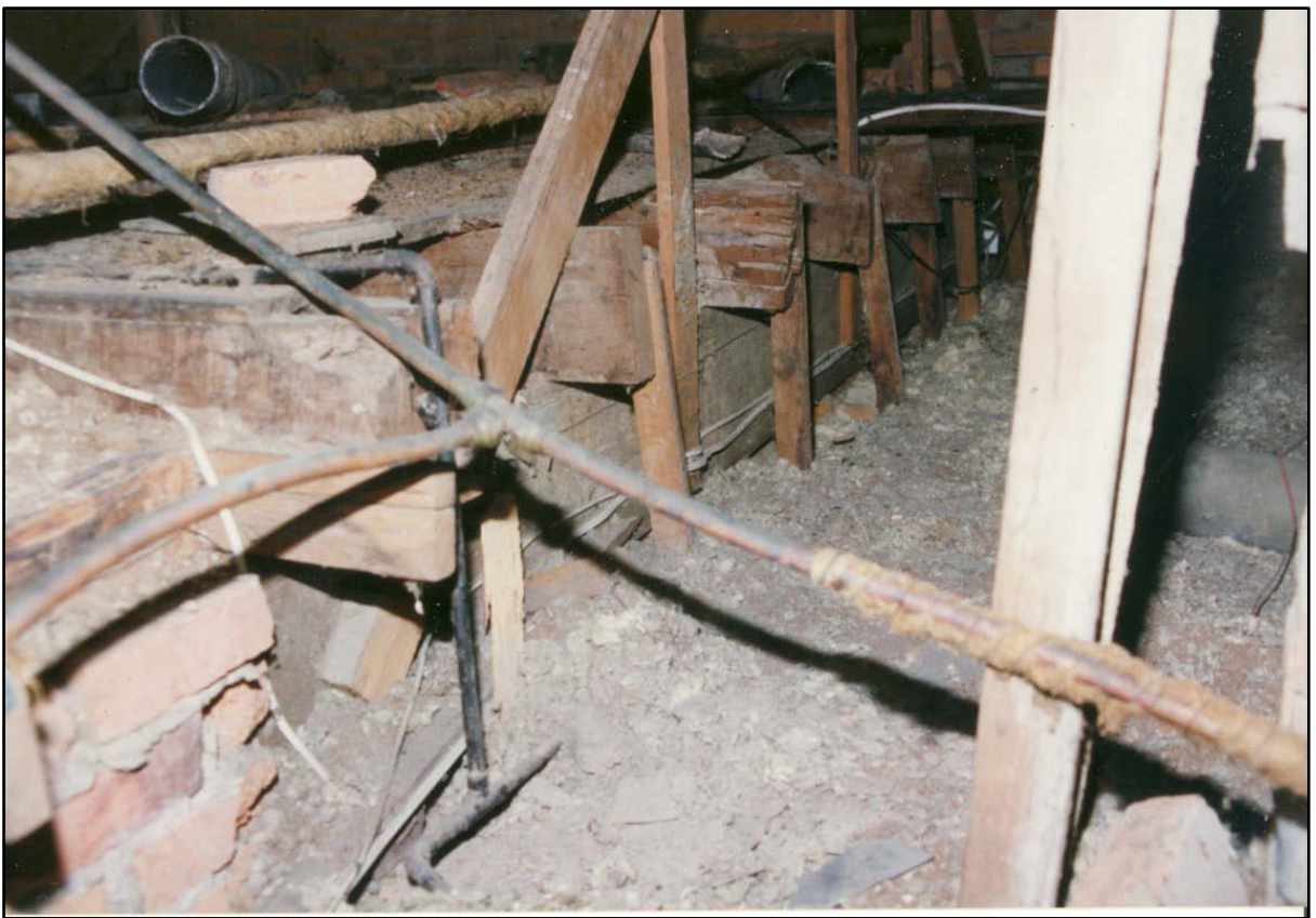
Photograph 69 Shown here are renovated ceiling joists in loft area, Culla Hill, with ceiling joists
