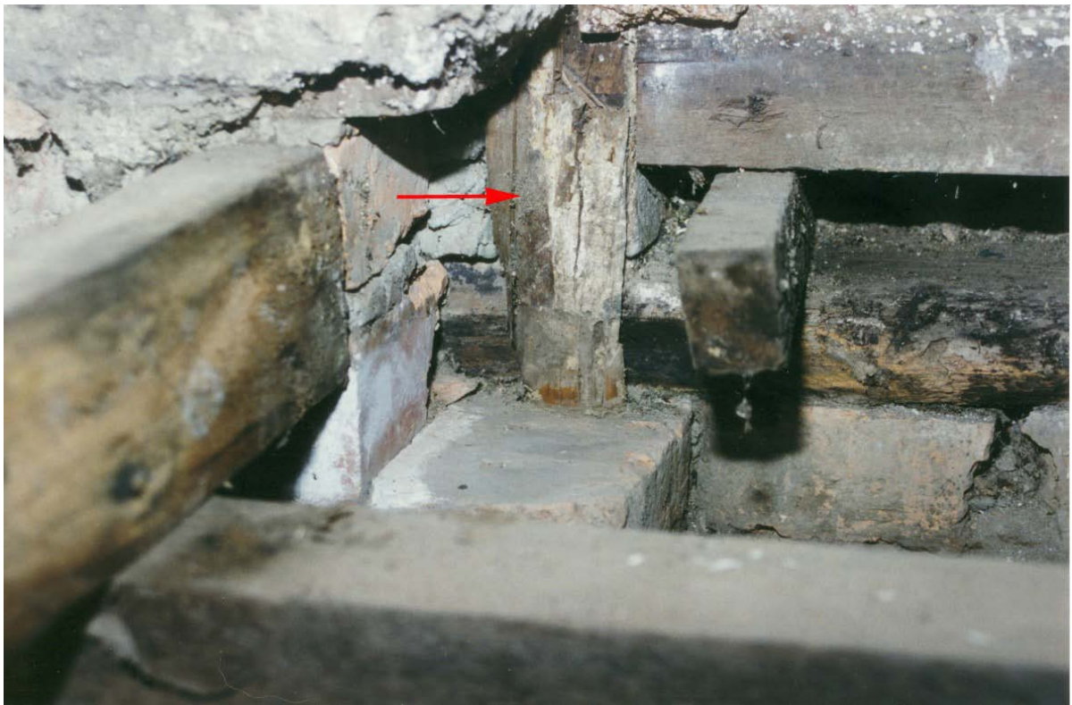
Photograph 15 Close up of architrave fragment, arrow, at original sill in internal door jamb, front door, Pontville homestead.
