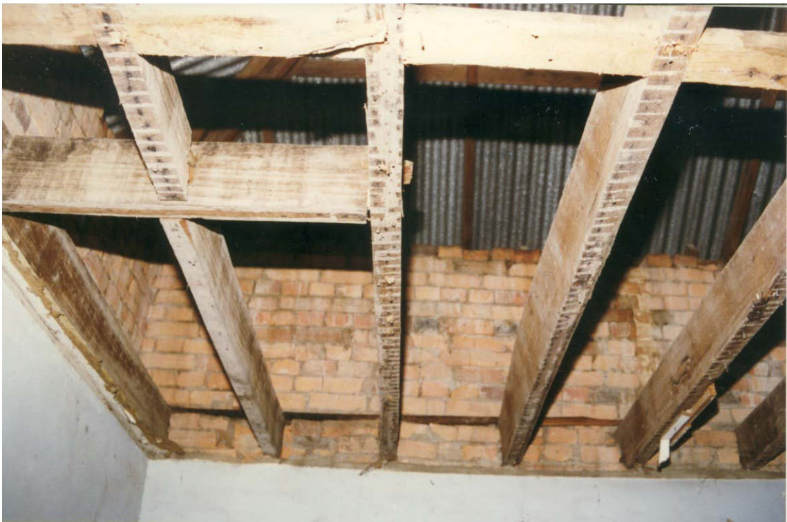
Photograph 11 Header beam and filler joist in loft opening, Pontville. Three shoulder and mortise joints are present in the beam and one of the tenons is fixed. Lath and plaster marks and nails are present on the underside of all joists, except the shorter joist that fills the former loft entrance.
