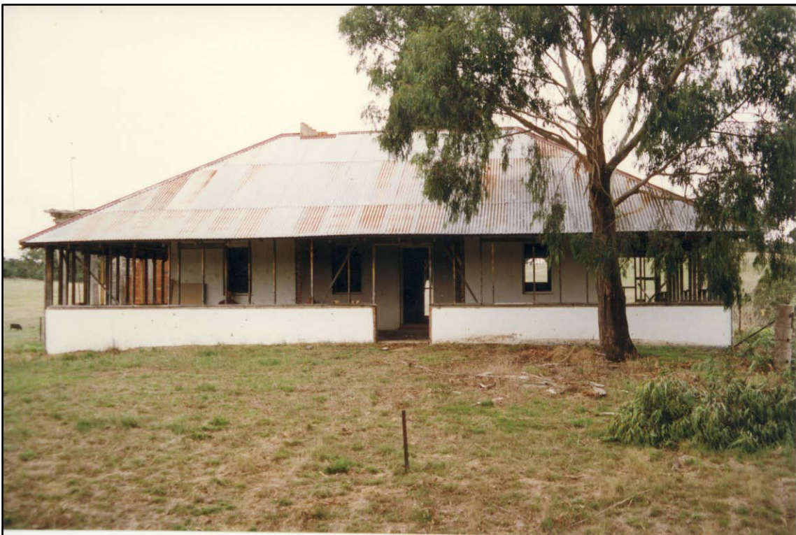
Photograph 7 Front of Pontville homestead facing Mullum Mullum Creek 1997. The front terrace can be seen in foreground and the roof seen here is a recent rescue to keep the weather out.
