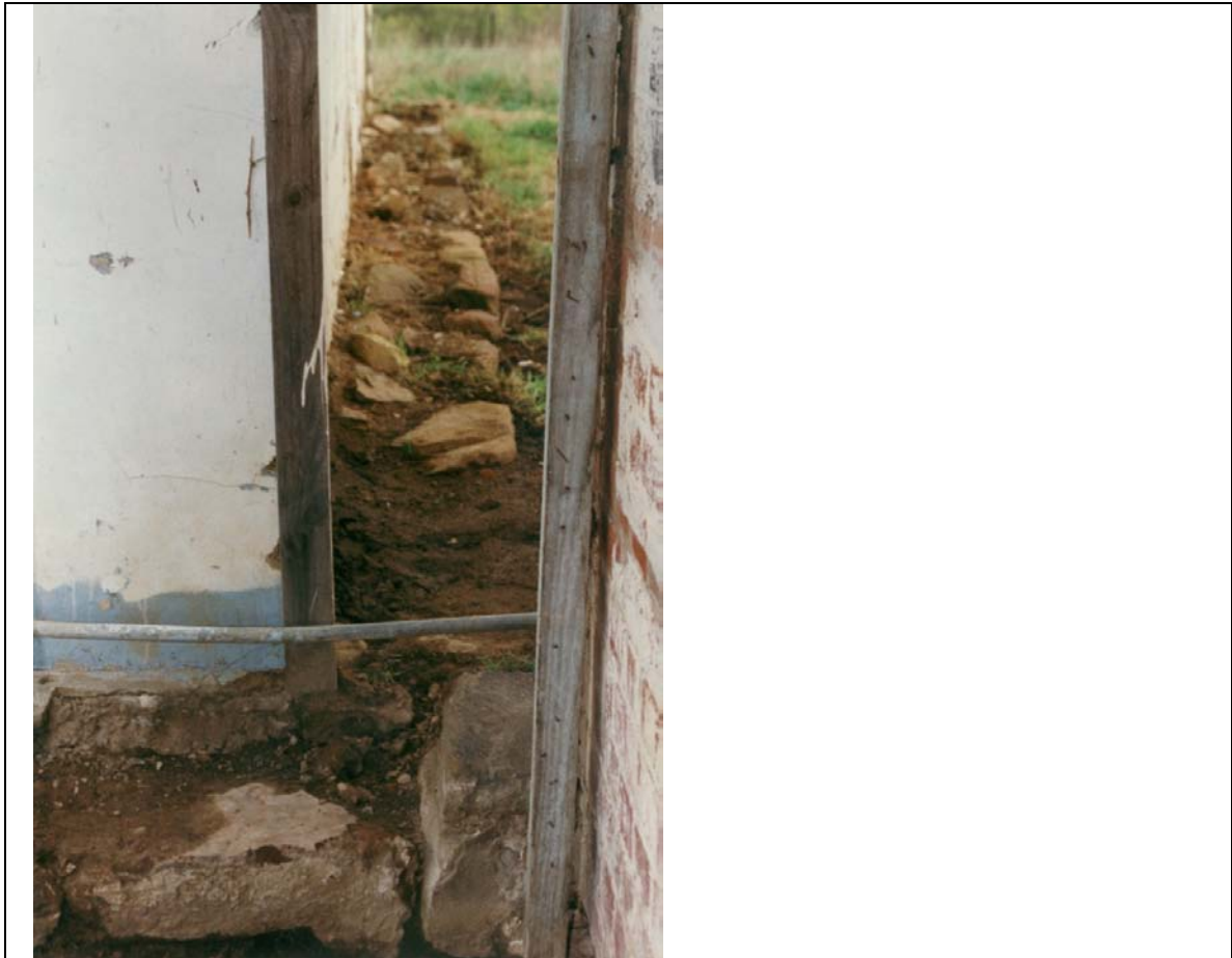
Photograph 45 Seen here is the original sandstone footing at the north wall abandoned in the 1950s renovation to enclose the north end room. This footing abuts the brick chimney base, right, and is visible outside the extant dwarf wall of the east verandah to the left.
