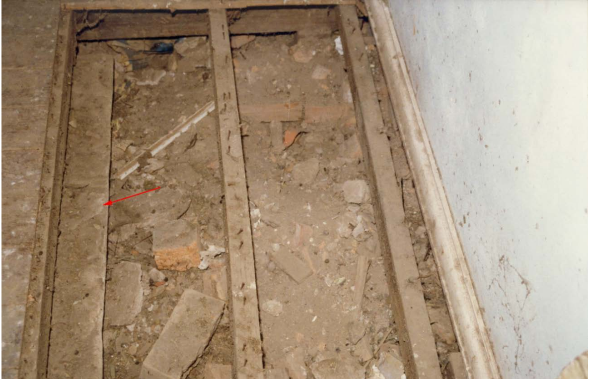
Photograph 18 Fireplace opening in south room with edge of sandstone hearth stone, arrow, beneath ex-tant floor. The stone marks the original floor height. The demolition material beneath this floor contains significant mid-19th century fabric.
