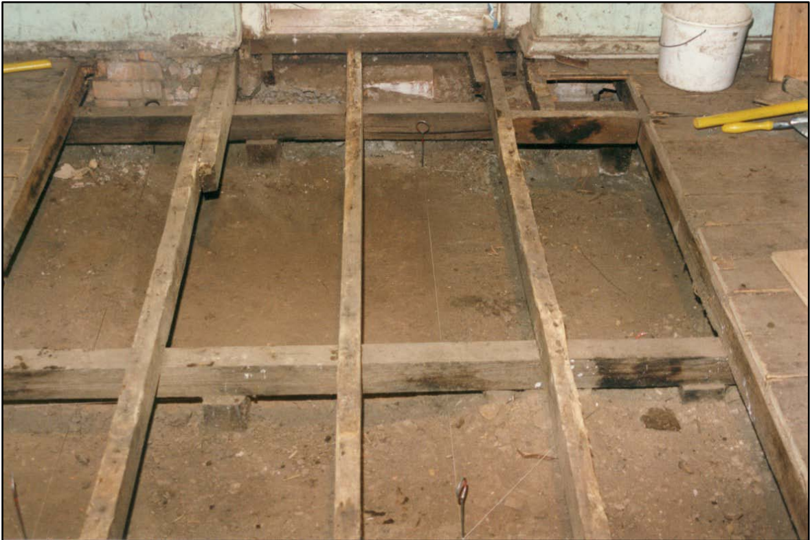
Photograph 14 This floor opening in the central room reveals sub-floor deposits excavated in this assessment. The string line marks the excavation area of Trench 5. Floor level is raised above original installed by Newman. Lower front door fabric is visible at top of photograph.
