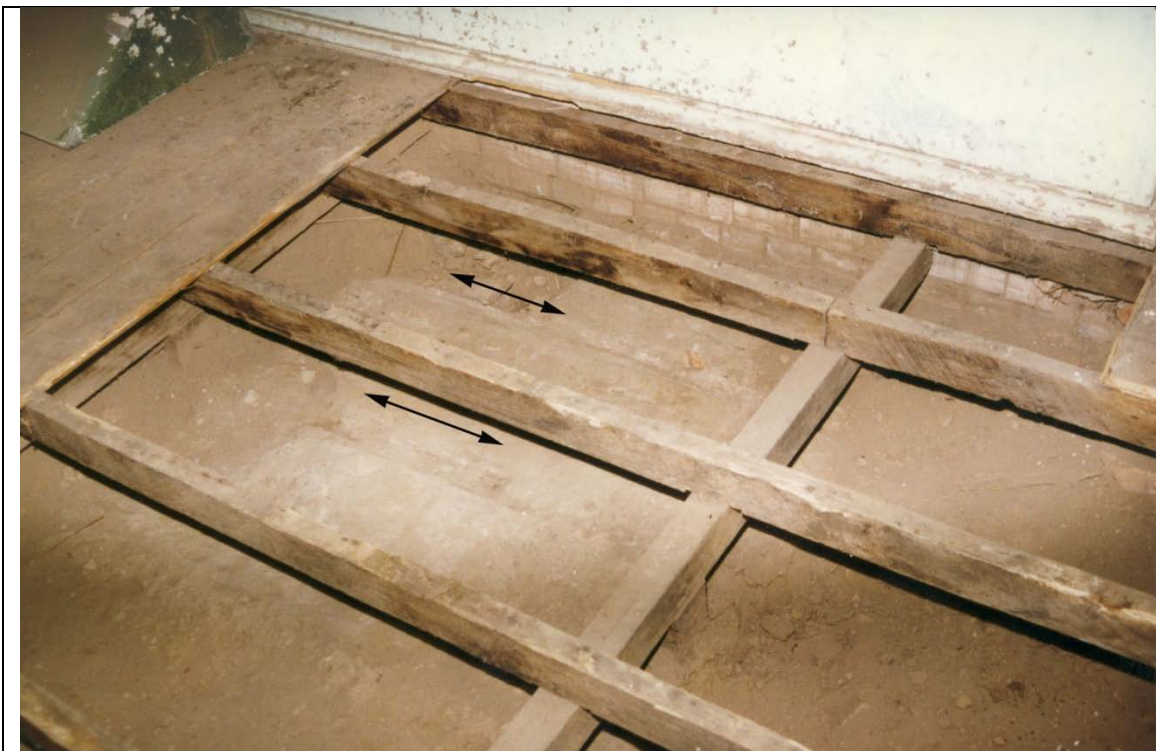
Photograph 60 Found in the sub-floor area of the central room of Pontville in Trench 5 is a weak mortar pad (seen as a light colour between joists) on which are parallel linear impressions, arrows, made by former floor joists. These marks occur outside Trench 5.
