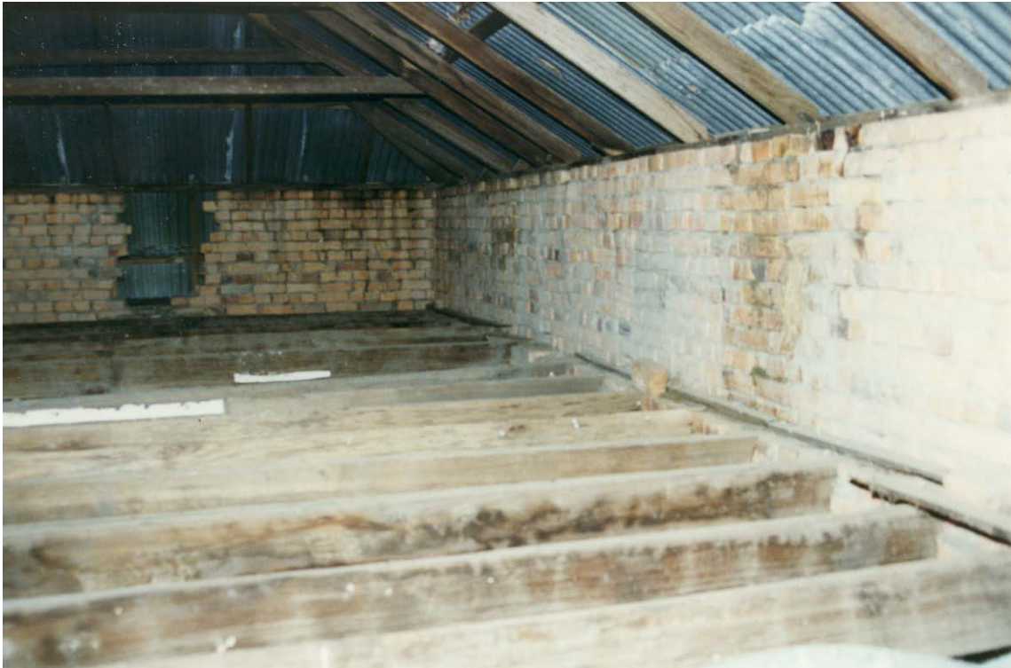
Photograph 10 Interior walls of loft. Slate, shingles, nails, and other fabric from former roof were found in crevices and ledges of the loft and in the sub-floor cavity below.
