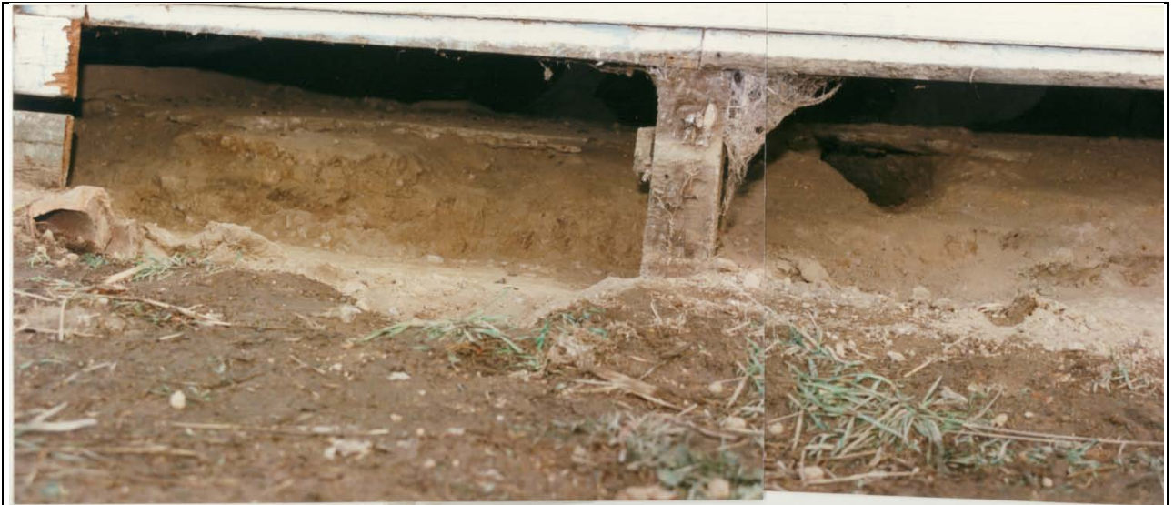
Photograph 57 Seen here under the raised timber floor of the east verandah is a thin mortar floor capping a layer of fill that may contain artefacts. This floor may be original. A thin concrete footing for the outside wall of the verandah, presumably a renovation that was not used, can be seen abutting the timber upright post. Trench 4. Composite image.
