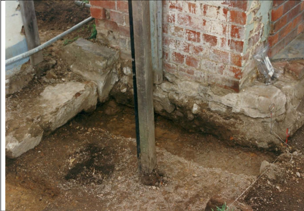
Photograph 49 Seen here is the fully excavated Trench 2 showing a large square post hole next to the vertical timber post and the junction between the stone footings of the chimney and home- stead (left).
