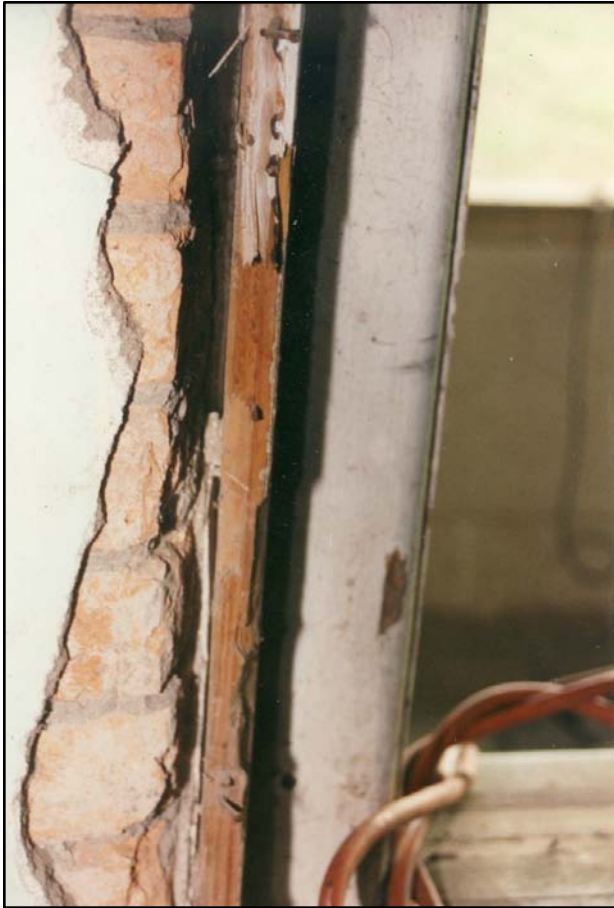
Photograph 20 Shown here is the timber window surround, beaded trimmer strip fragments, and attachment nails, with hand-made bricks exposed behind a renovation plaster.
