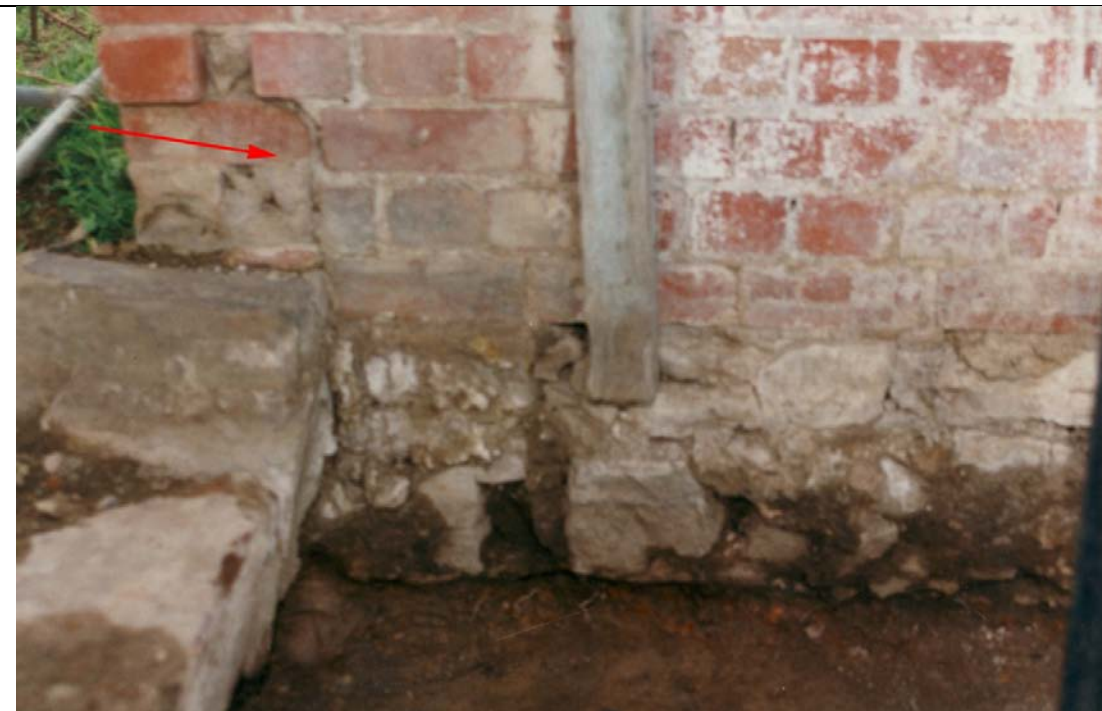
Photograph 48 Recess in brick work (arrow) indicates homestead stone footing on left was built first and that its upper coarse is missing. Trench 2 showing base of chimney footing.
